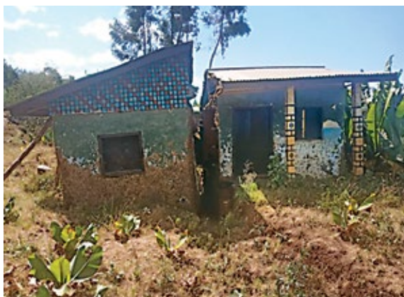
Figure 7-5. Building destroyed by an active landslide, Widesa.
