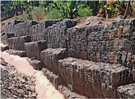
Figure 7-6. Tilted gabions in an active landslide in the main road, south of Yirga Chefe.
