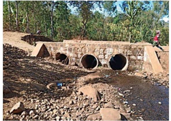
Figure 7-7. Culvert with insufficient width and limiting run-off capacity of the stream.
