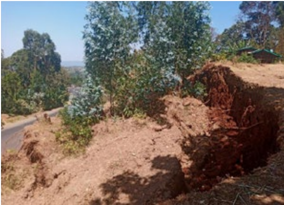
Figure 7-2. Shallow landslide in the roadcut formed by completely weathered basalts.
