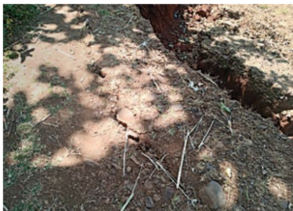
Figure 7-4. Tension crack of active landslide close to main road between Yirga Chefe and Gedeb.
