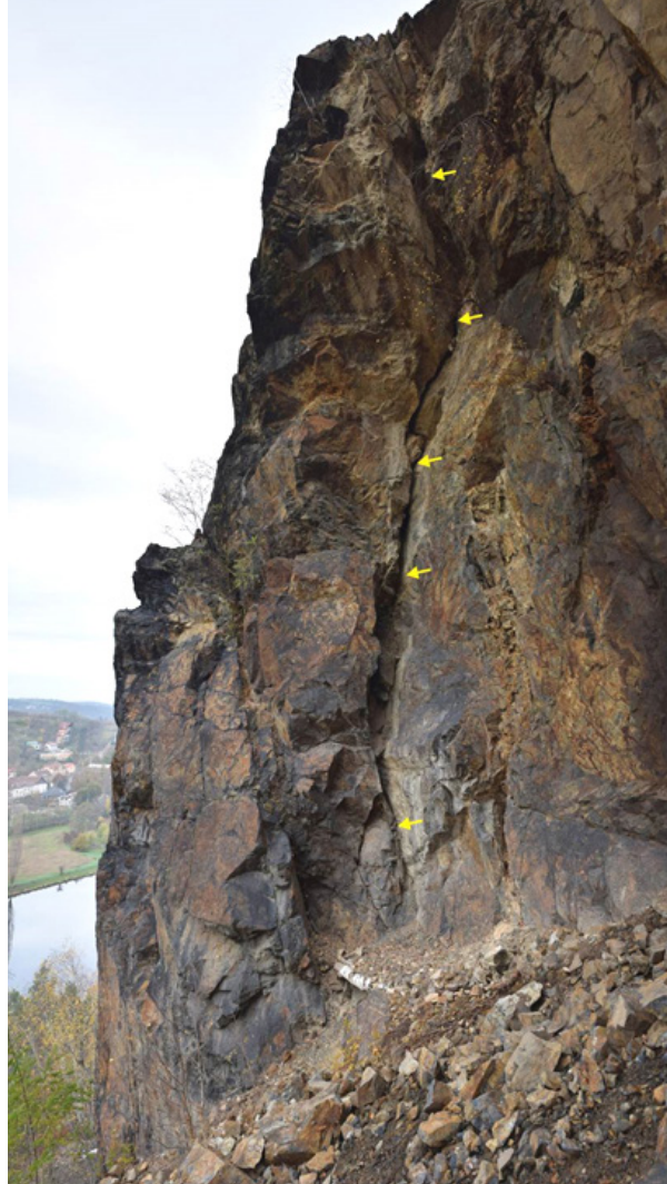
► A general view of the detached rock pillar in the northern vicinity of an existing main scarp in the Větrušická rokle National Nature Reserve. A continuous vertical fracture is highlighted by yellow arrows.
