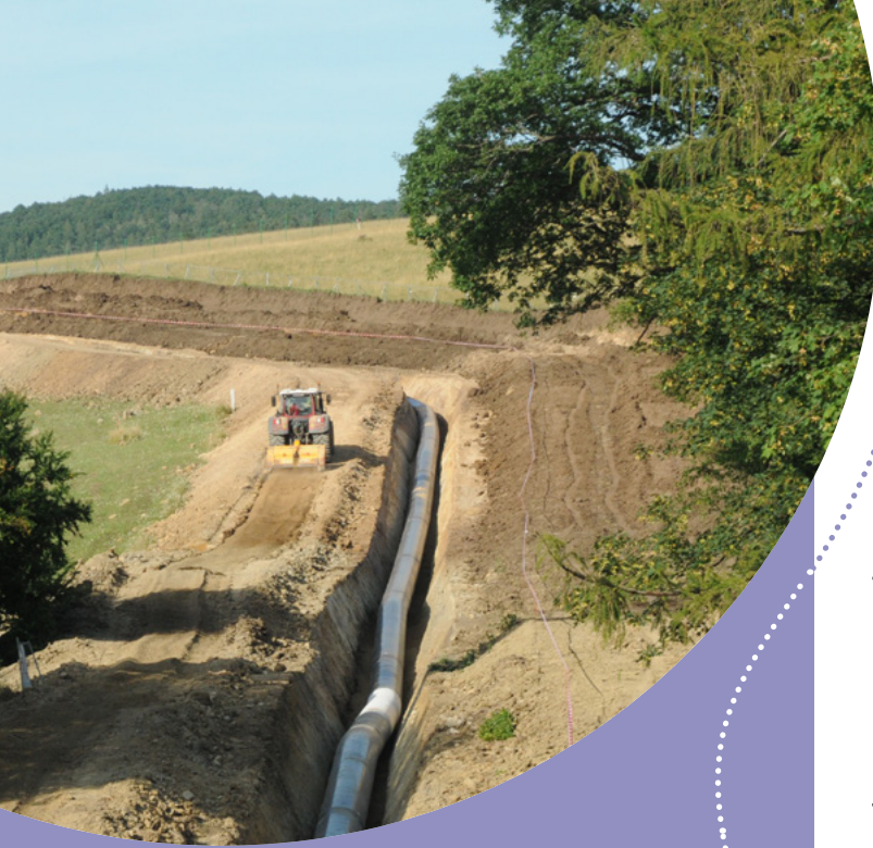
► Slope deformation 24-44-18/3 with a Moravia gas pipeline in Jestřabice. Photo by O. Krejčí.
